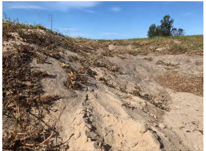
Looking with the camera placed on the top of the concrete at the outlet looking out (west)
